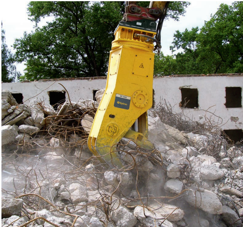
The Bulk Pulverizers' smart design also makes them ideal for primary demolition of ceilings and walls.
